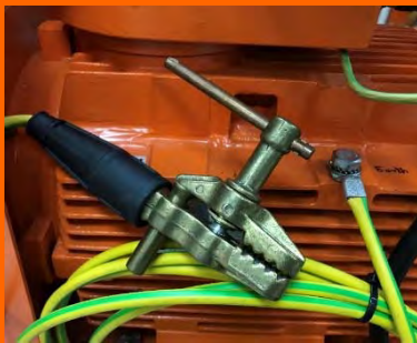
Earth Cable with Clamp.
