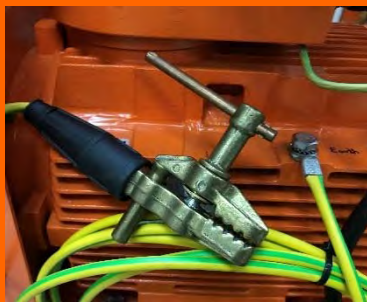
Earth Cable with Clamp.
