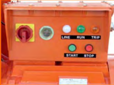
Electrical box with main switch, overload relay & hour meter.
