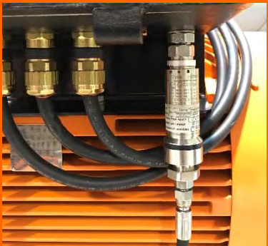
Cut-off switch for low inlet water
